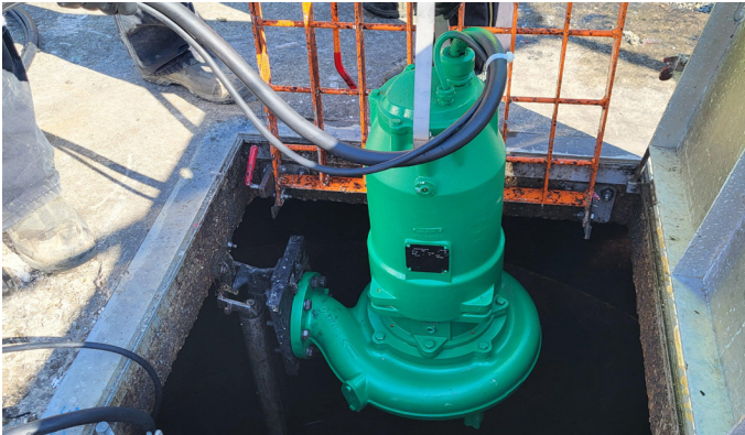
The Pentair Hydromatic Next-Gen Submersible pump is lowered into the wet well at County Home Lift Station.
