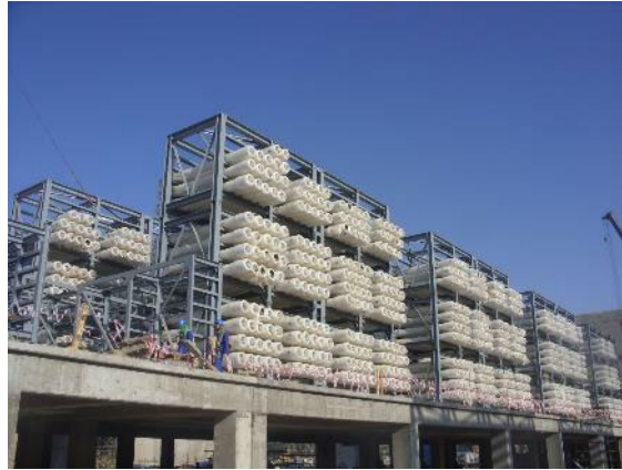
PROJECT SWRO III Capacity – 240,000 m 3 /day No. of Codeline pressure vessels: : 11" – 3616 / 8" - 848
